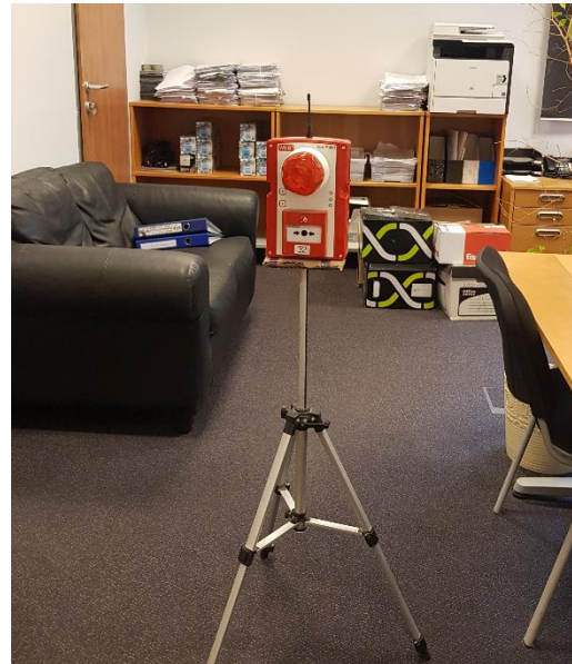
Figure 5. Used fire alarm sounder, source: own photo
