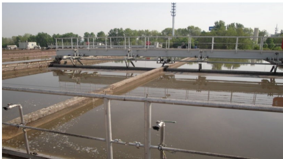
Figure 1. Rectangular settling basin
