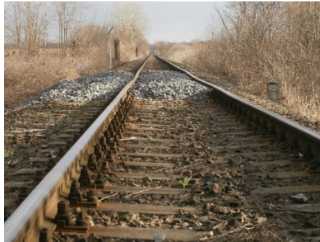
Figure 12. Local substructure failure [32]
