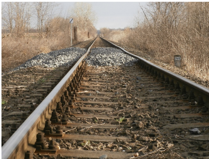
Figure 6. Local substructure fault due to cavity rupture [21]
