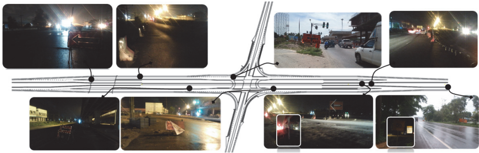
Figure 6. Traffic signs and road marking issues
